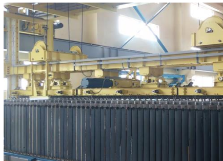
Figure 1. Gantry crane for CE
