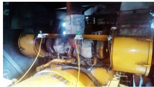
Fig. 12. Example of working transmitters units installed on engine
